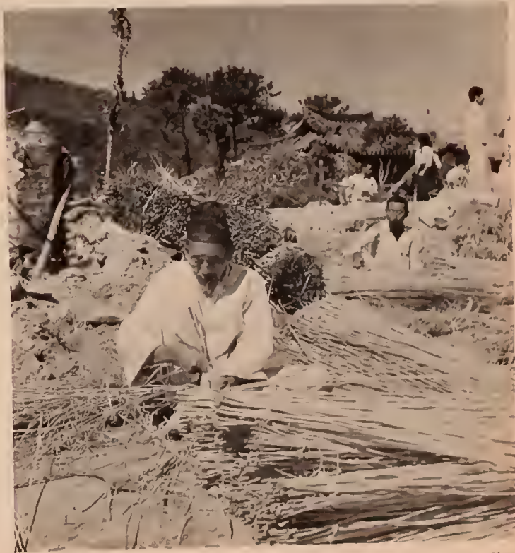
Chinju, 60 per cent destroyed in 1950, is being rebuilt by resilient Koreans. Here workmen, using available material, weave bamboo to form the roof of a new house.
